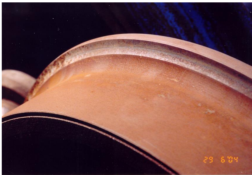
Figure 4 - An unacceptable witness mark
