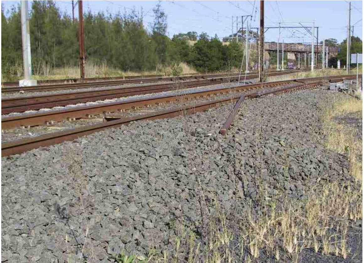
Figure 3 - Example of catchpoint with poor landing zone
